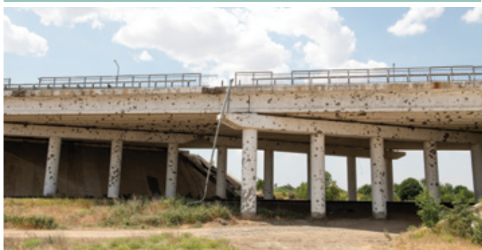
A bridge near the border between Kherson and Mykolaiv oblasts, Ukraine, damaged by a cluster munition strike. Bridges and other critical transportation infrastructure are often targeted.
